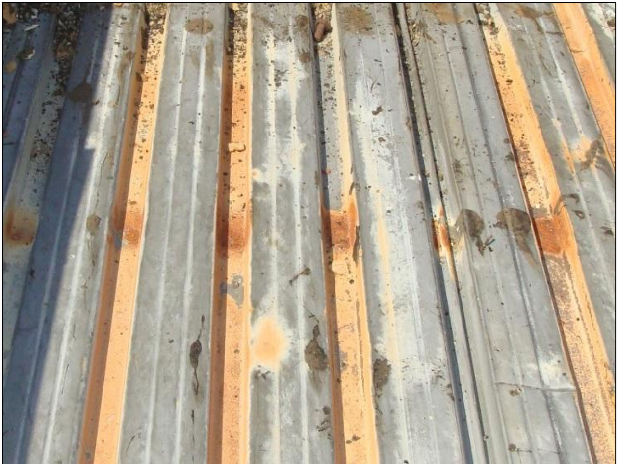
Photo of Level 2: Light to Moderate Corrosion
