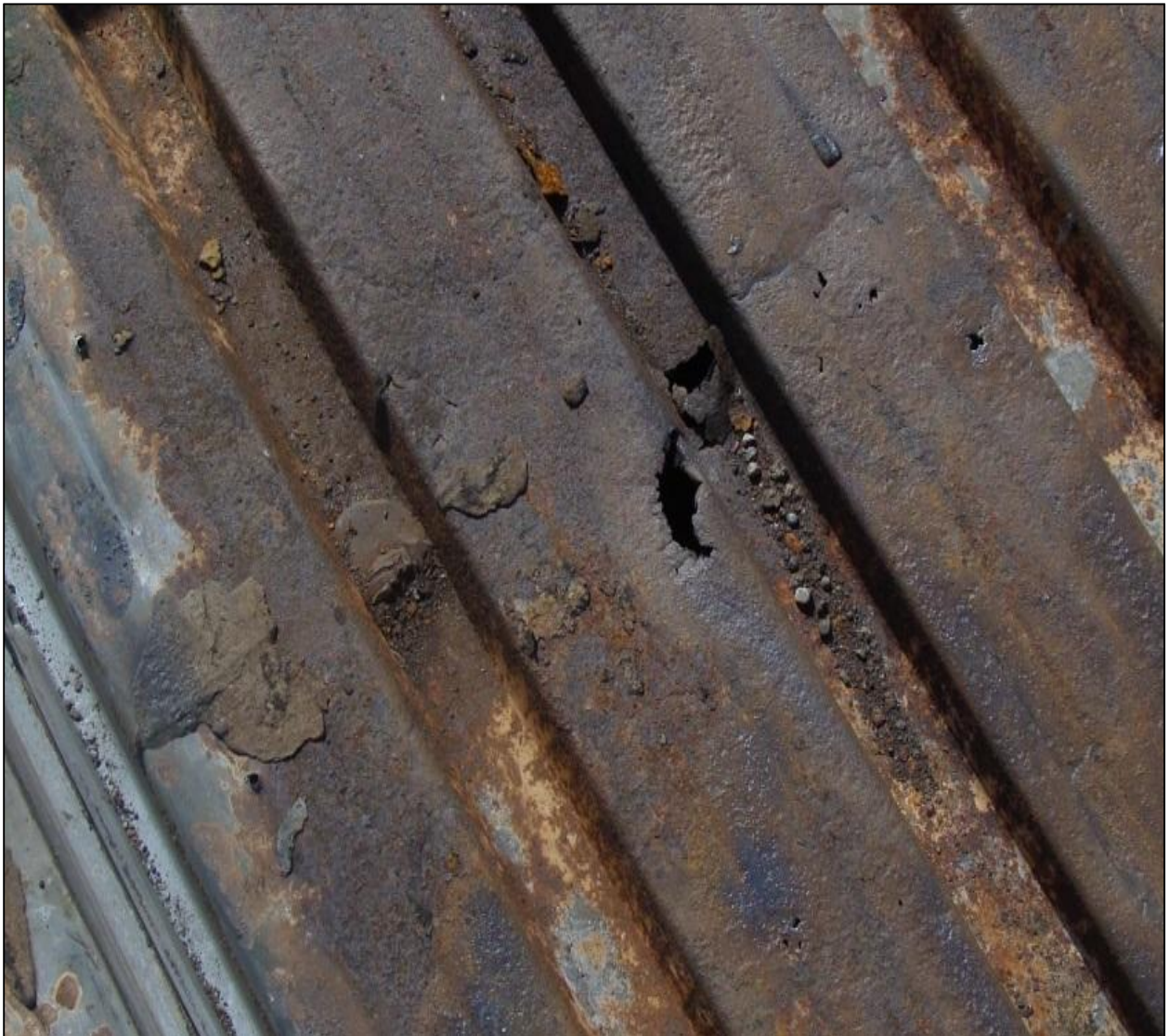
Photo of Level 4: Severe Corrosion With Holes
